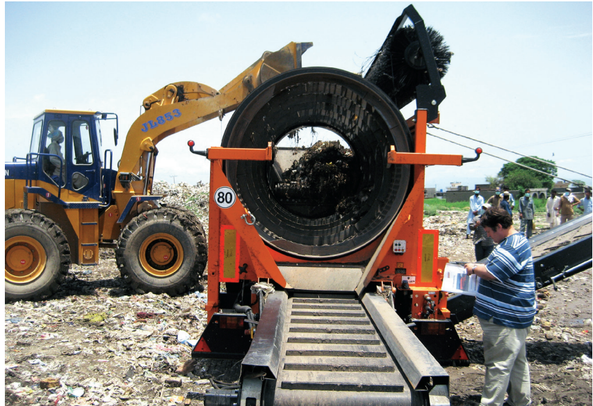
The process of recycling the waste.
